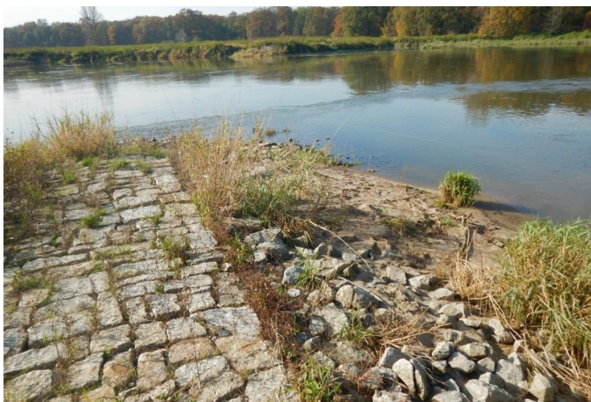
Pic. 1 Restoration of vegetation and sandy bar on one of the groynes reconstructed in 2012-2015
