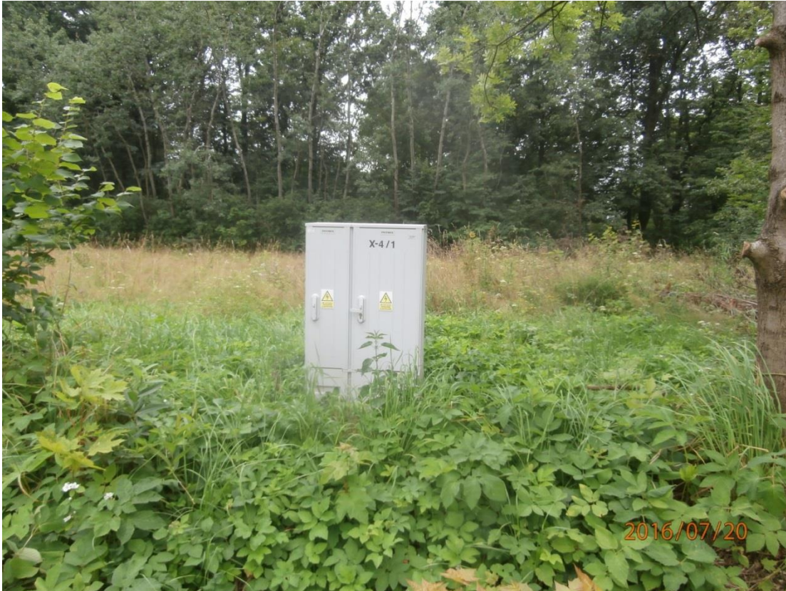
Figure 6 –View from the existing district road No. 3233D on the plot No. 240 (indented disassembly of power infrastructure)
